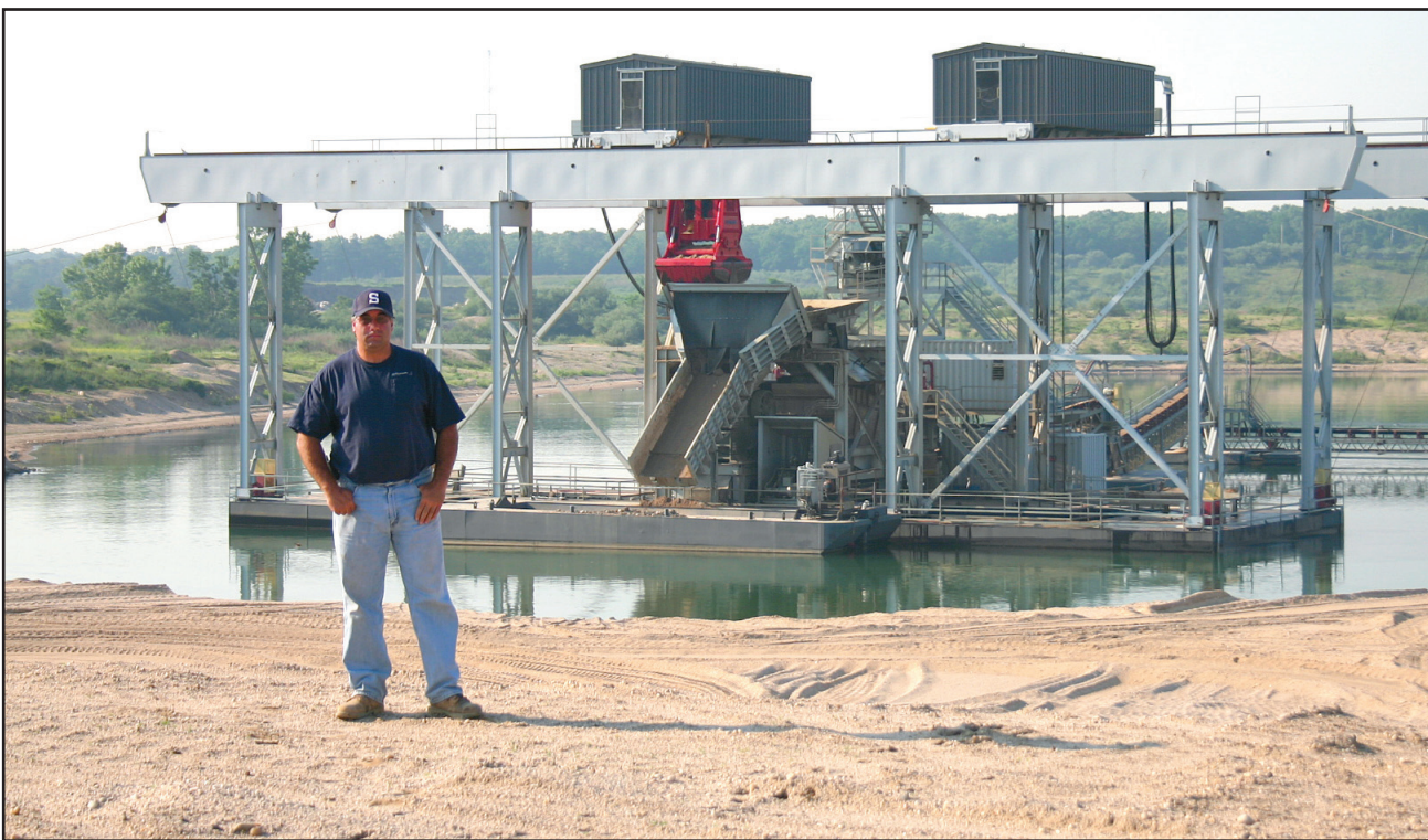
Mike Vigliarolo, vice president of Coram Materials Corp., with the twin 13-yard dredge, which consists of two 8-foot X 20-foot primary screens, two 40-ton trolley cranes and a pair of 13-yard spade-nosed buckets.
