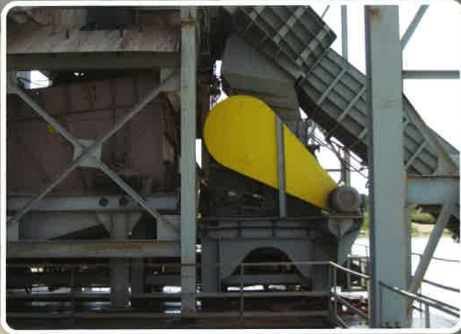
SCREEN, CRUSHER & OVERSIZE CHUTE
