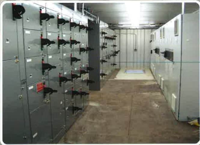
ELECTRICAL CONTROL ROOM
