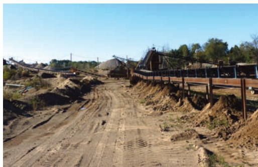
Mined material is conveyed overland to the primary screen plant on the right. From there, material moves on to the McLanahan Lites-Out classifier in the distance on the left.
