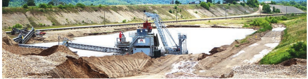
Jaymar’s dredging operation from atop the pit. The top of the screen plant can be seen in the distance over the far berm, just to the left of the abandoned farm structure and tree.
